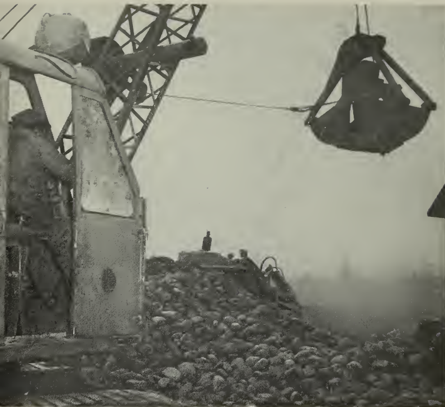
CLEARING THE WAY —Many skills are needed in the construction of a Navy base. Here, equipment operators clear the way for other ABC men to move in.
